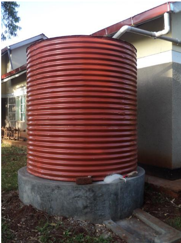
Figure 6: The newly installed gutters and water tank for water storage and supply during scarcity/rationing.
