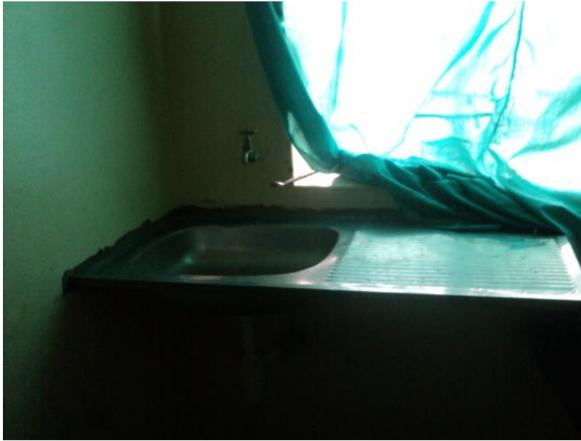
Figure 7: One of the three water sinks connected in the building
